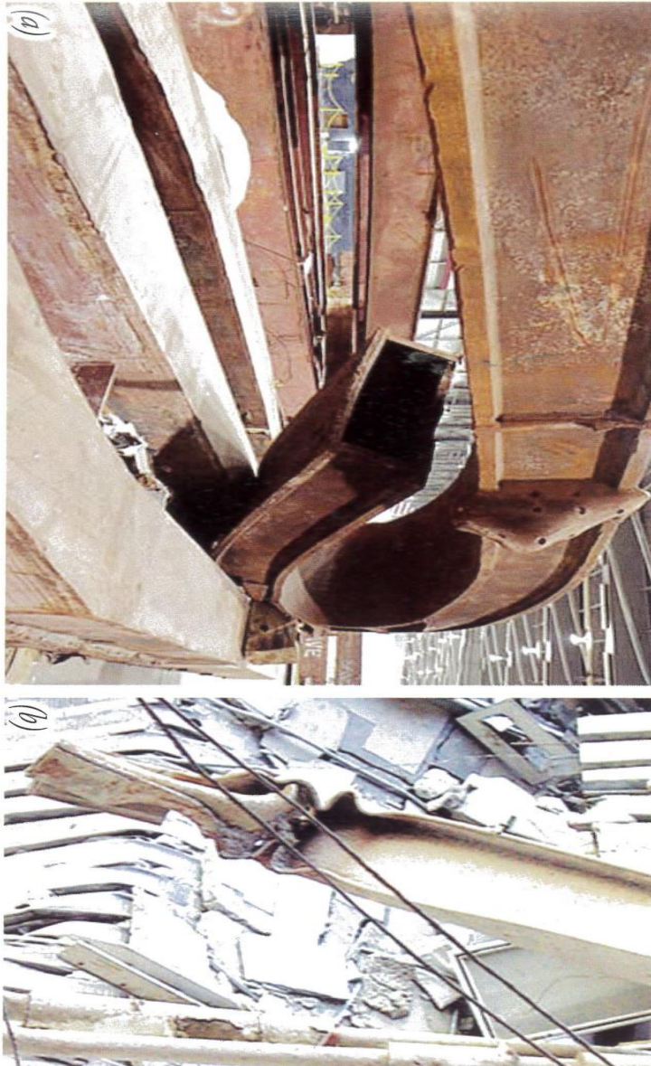
Figure 370. (a) WTC core column curled, not buckled. A gravity-driven "collapse" would not do this. The beam above has smooth curves, without kinks. (b) This beam shranked up and has see-through holes in it,
