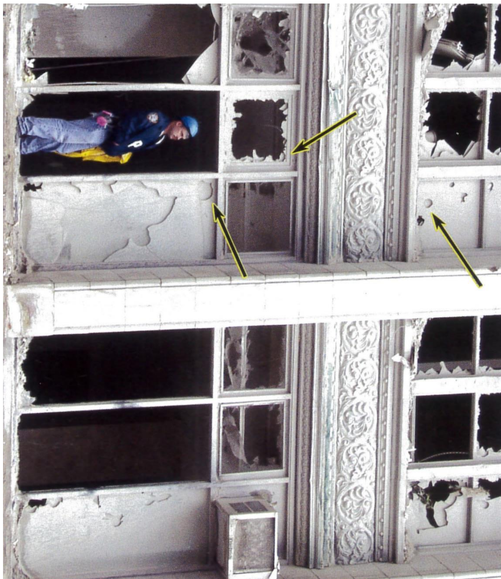
Figure 5 strange broken double planed windows
